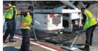
PRESSURE WASHING & RECLAMATION
