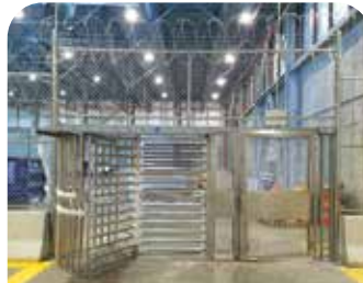
Access Control Systems JFK Airport
